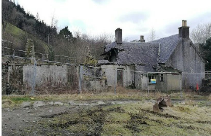
Unit three (left) and unit one (right)
